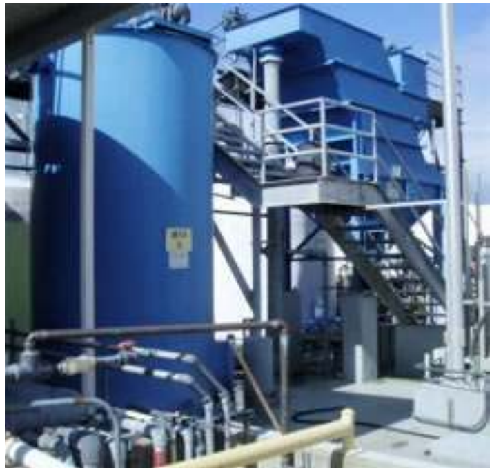
Packaged Industrial Wastewater Treatment Plant Illawarra, NSW
